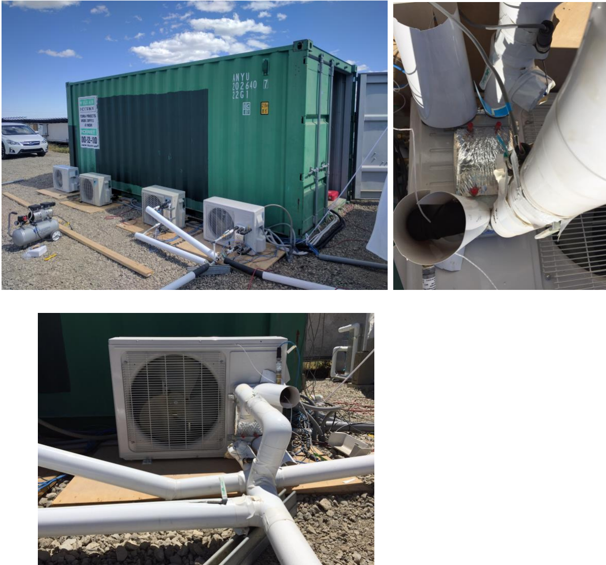
Figure 3: Picture of the exterior of the container space cooled by the A/C units and the modified A/C units
